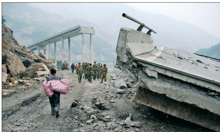
A collapsed section of the elevated expressway near Yingxiu Town, Wenchuan County
