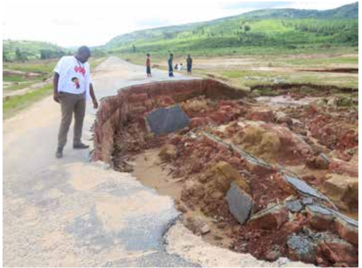
MSF Emergency Coordinator assesses a damaged road in Chimanimani
